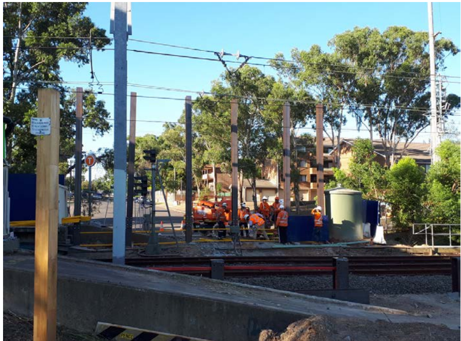
Image of post installation for hoarding undertaken at Kingswood Station during the recent track-work shutdown
